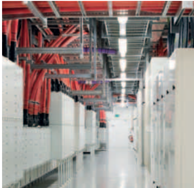
Chilled out: inside Global Switch's London II data centre in East India Dock, E14, where rooms are kept super-cool
